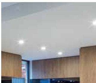
Led Lighting Internally
