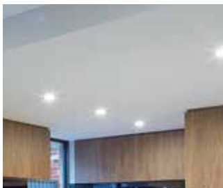
Led Lighting Internally
